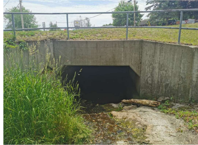
Good Condition Inlet Components
