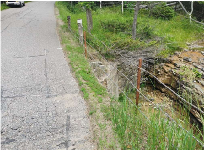
Poor Condition Guiderail
