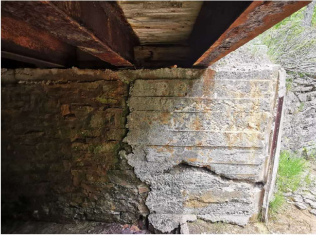
Fair Condition Abutment Wall Extension
