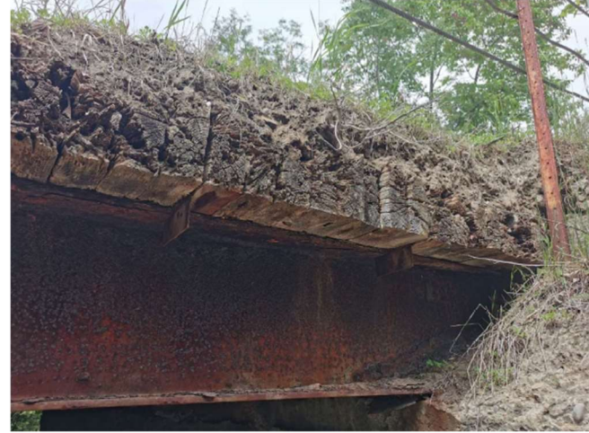
Poor Condition Deck
